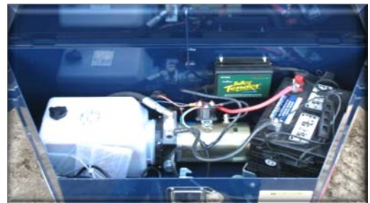
Pump & battery box, w/ optional battery tender
