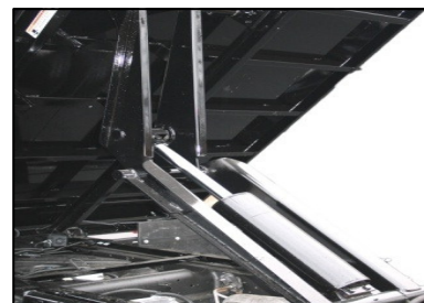
Champion Hoist, Installed
